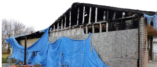
Fire destroyed the roof and garage
